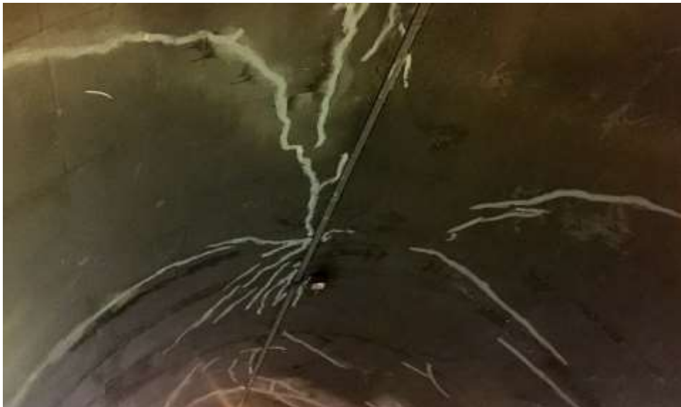
Photo 4-54 View of Recently Generated Joints in Tunnel-2.
