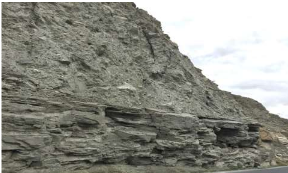
Photo 4-68 Development of Jointing in ABGM Underlain by Rock along KKH.
