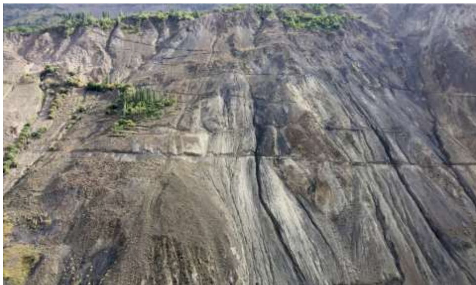
Photo 4-83 Highly Crushed Rock in Maicher Village along Road.
