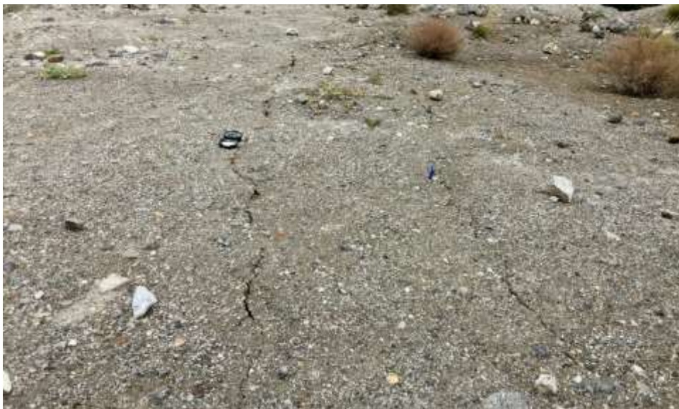
Photo 4-60 Development of Parallel Joints near SCO Building.
